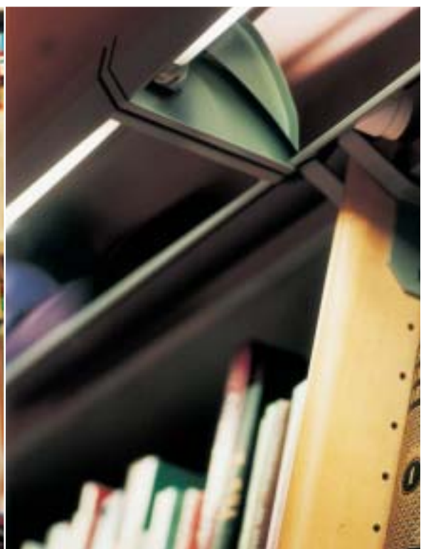
▲ Each bay is fitted with Eurobib's light fixture, "Eyeline", allowing the general lighting to be dimmed.
